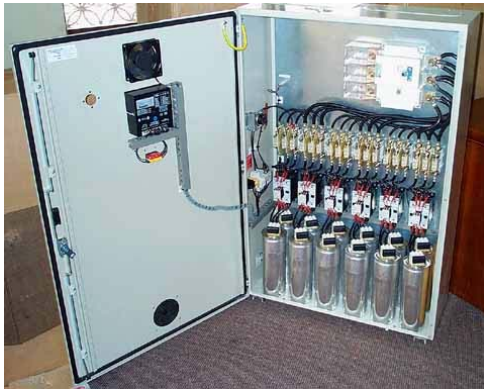
Automatic Capacitor Banks in a Metal Case
