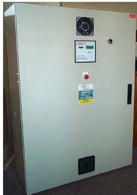
Metal Case containing Automatic Capacitor Banks
